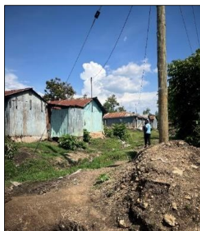
Figure 26: Electric pole in Shauri Yako affected by erosion (©SUEZ Consulting, 2025)
