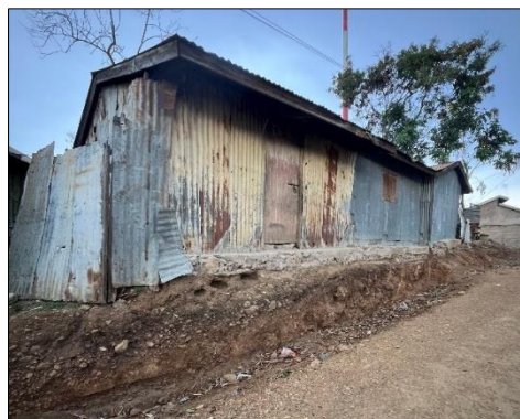
Figure 33: House at risk due to visible landslide impacts in Makongeni settlement (©SUEZ Consulting, 2025)
