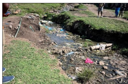
Figure 25: Photo of a water pipeline in the middle of the flood path surrounded by waste in Shauri Yako (©SUEZ Consulting, 2025)
