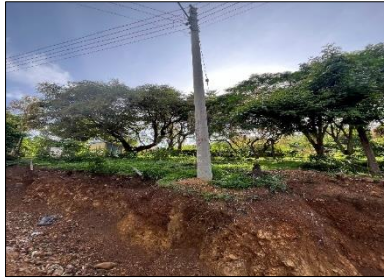
Figure 35: Electric pole at risk due to visible landslide impacts in Makongeni (©SUEZ Consulting, 2025)
