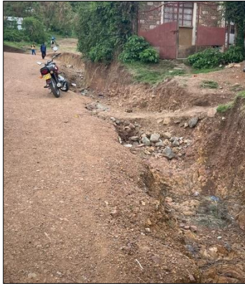
Figure 14: Important erosion on the side of the road – Makongeni settlement (SUEZ Consulting, 2025)
