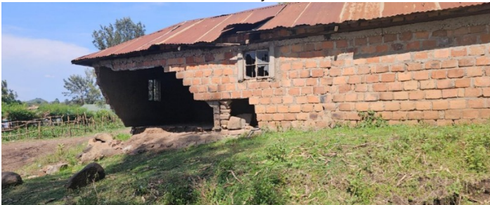
Photo 4: State of a Building in Sofia
